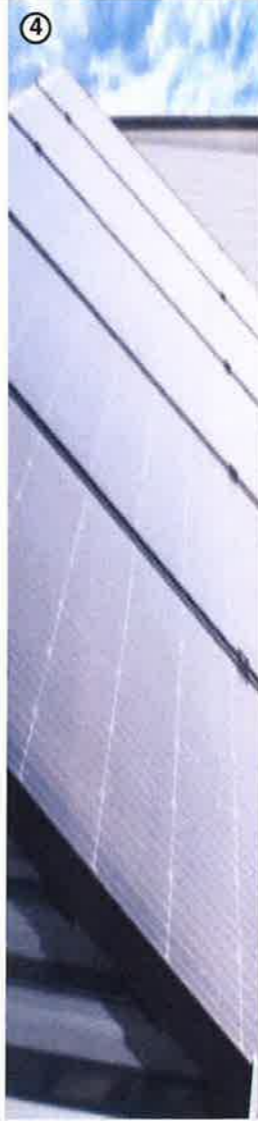
SOLAR COLLECTORS TO ROOF
