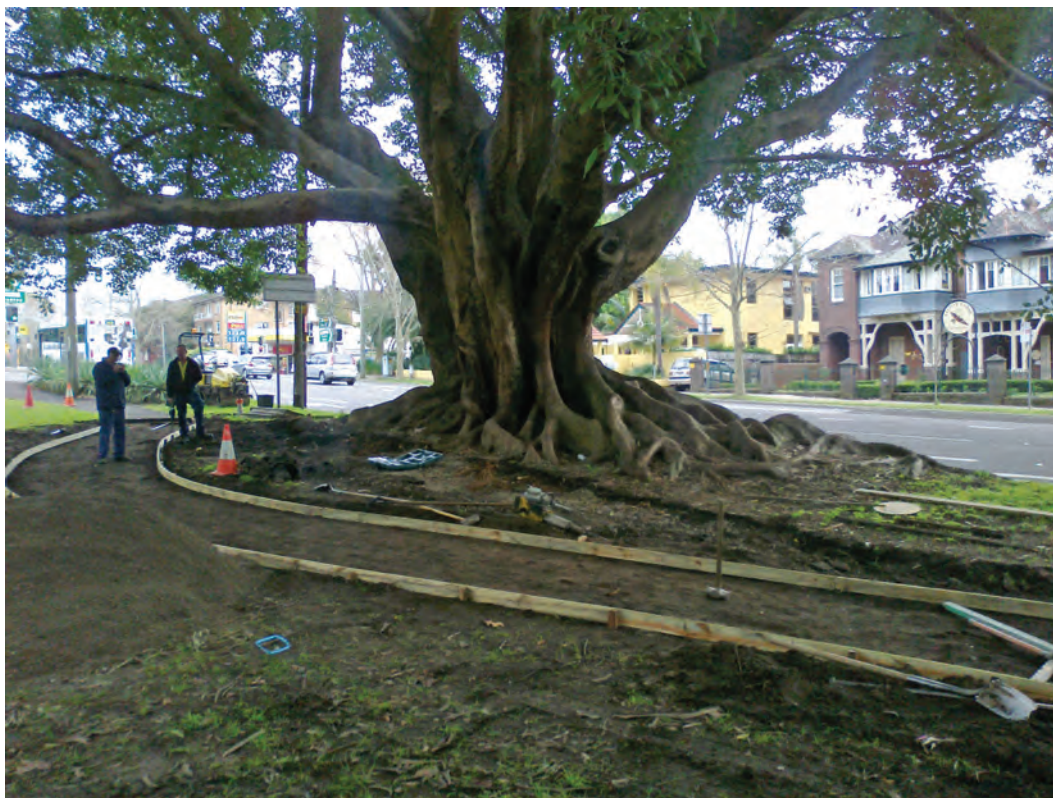
Footpath realignment around a significant Fig tree in St Leonards Park allows room for roots to grow without creating trip hazards in the new footpath.
