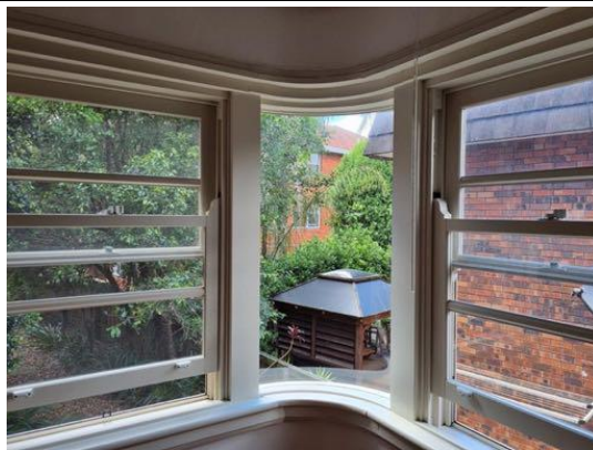
FIGURE 10: Curved glass to corner, with typical timber framed double hung windows with horizontal glazing bars to either side.
