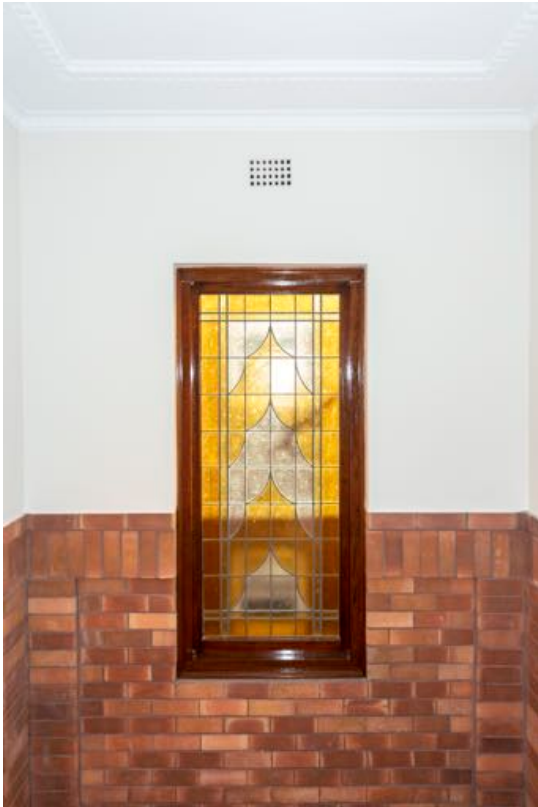
Figure 22: (Left) Leadlight window and original plaster ceiling with decorative cornices to stair lobby.
