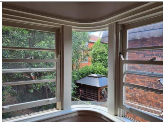
FIGURE 9: Curved glass to corner, with typical timber framed double hung windows with horizontal glazing bars to either side.
