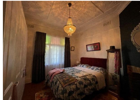
Figure 5.55 First floor apartment to west— bedroom with original plaster ceiling and stained glass timber-framed windows.
