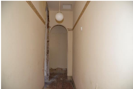
Figure 5.72 View of the central hallway with some intact original Victorian wallpaper. stripped.
