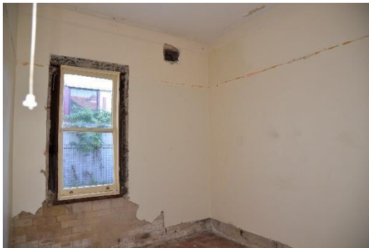
Figure 5.74 View of a room with its Victorian features—the ceiling vents and window architraves—stripped. cornices—stripped.
