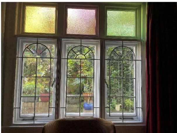
Figure 5.56 First floor apartment to west— original timber-framed casement windows with stained glass.
