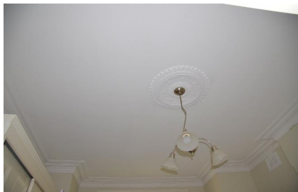
Figure 5.22 View of the plaster cornices and ceiling rose to the front bedroom.
