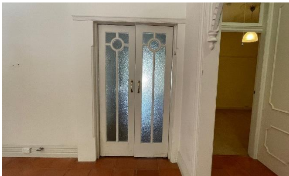
Figure 5.37 View to an internal door with stop living chamfering detailing along the doorway.
