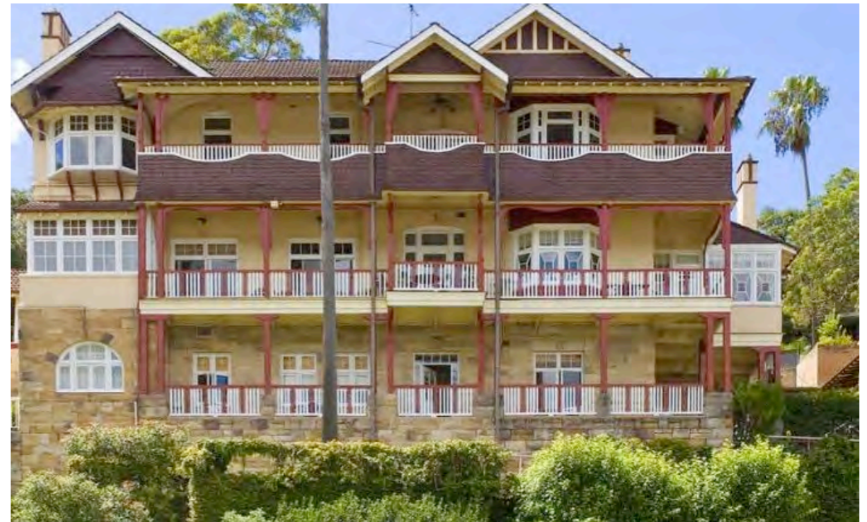
3. Painted timber fretwork to existing balconies - refer to colour schedule for paint selection
