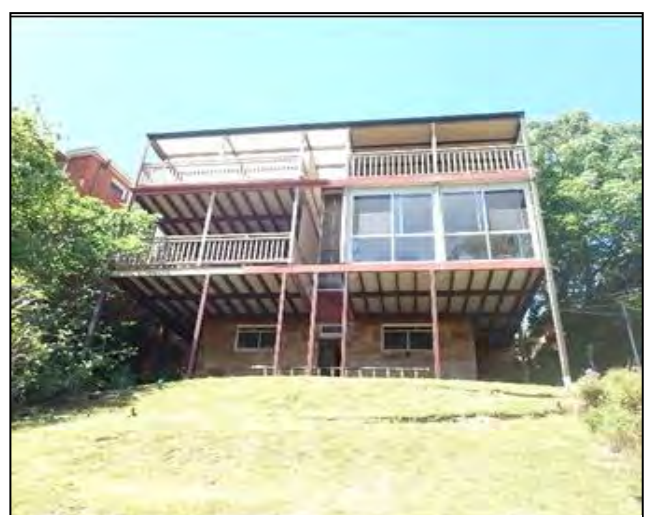
Figure 8. View of the rear of the subject site, showing the existing balcony structure.
