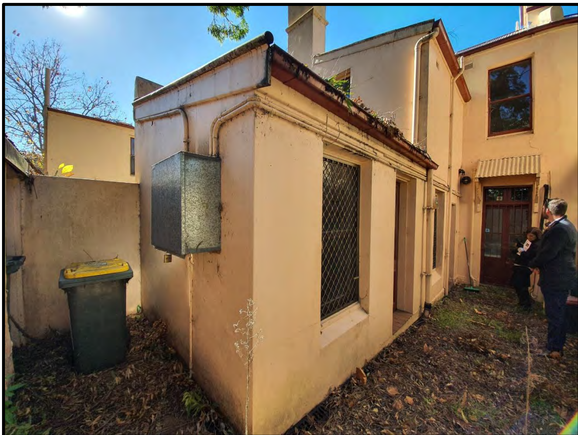
Figure 10: Old soil room, left of food preparation room, proposed timber deck (right) in rear
