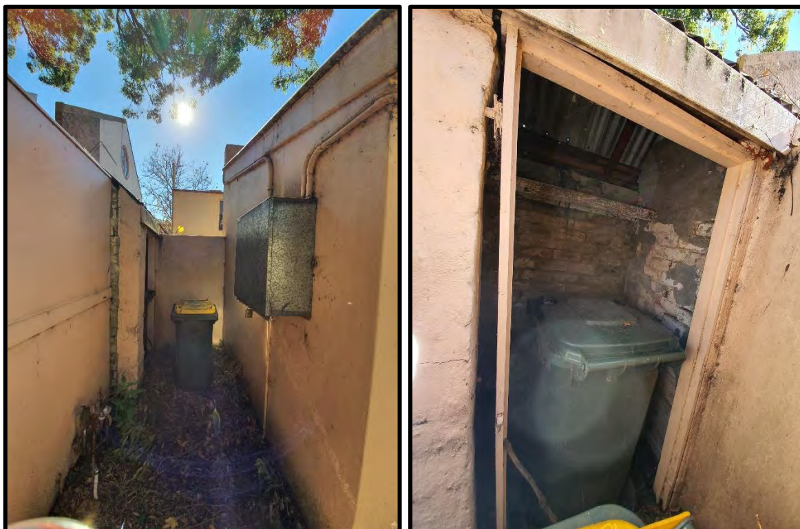
Figure 2 (left): View towards soil room, proposed solar battery unit inverter above switchboard (right)
