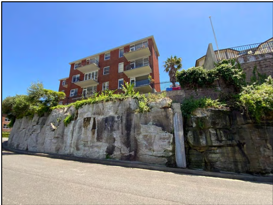
Figure 24: Southern side of existing building and rock wall – viewed from Henry Lawson Avenue
