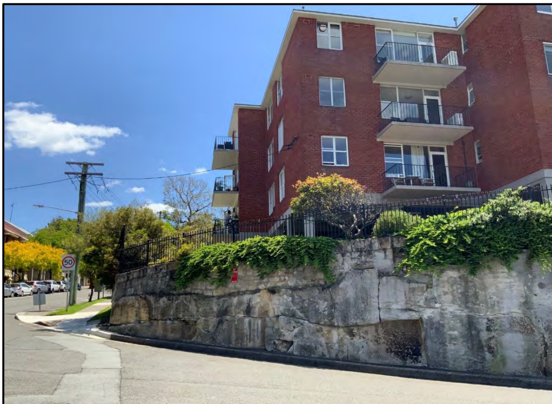
Figure 25: South-western side of existing building and rock wall – viewed from Henry Lawson Avenue
