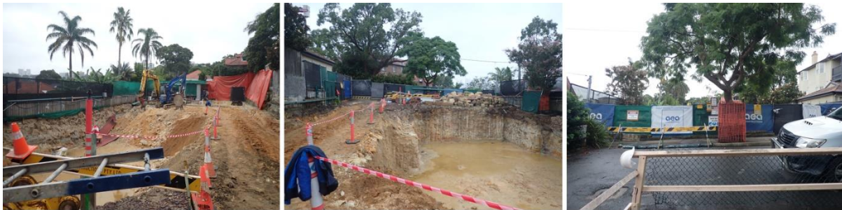
Figure 7 – Photos of site subject to demolition and earthworks and photo from street (North Sydney Council, 24 March 2022)
