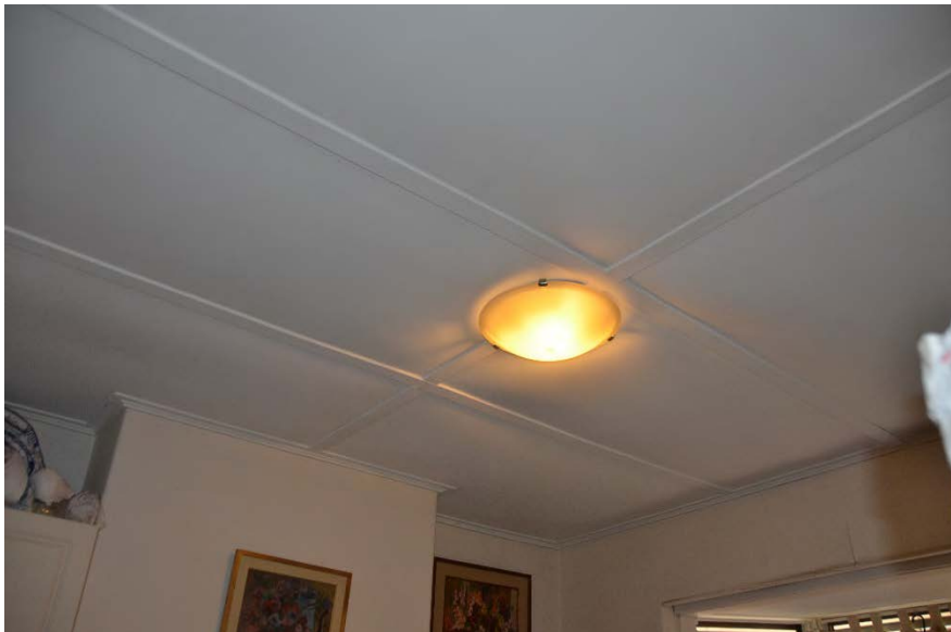
Figure 5.4.14: Front Bedroom showing replaced ceiling, batted joints, simple cornice and modern fitting.
