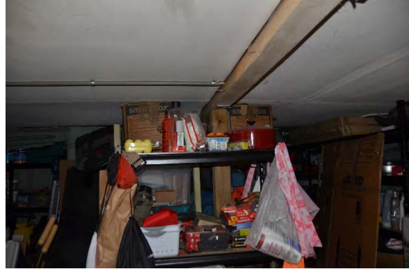
Figure 5.4.30: Lower Ground laundry area. Space with concrete slab and plastered lined ceiling. Recent prop in the centre of the room to support the floor structure.
