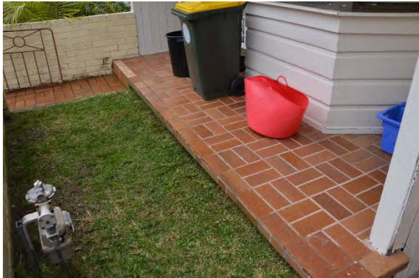
Figure 5.4.3: Original front timber porch replaced with concrete slab and tiles.
