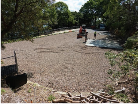
Caption: Bushcare Community Nursery, concrete slabs poured for sheds and shelter, March 2011.
