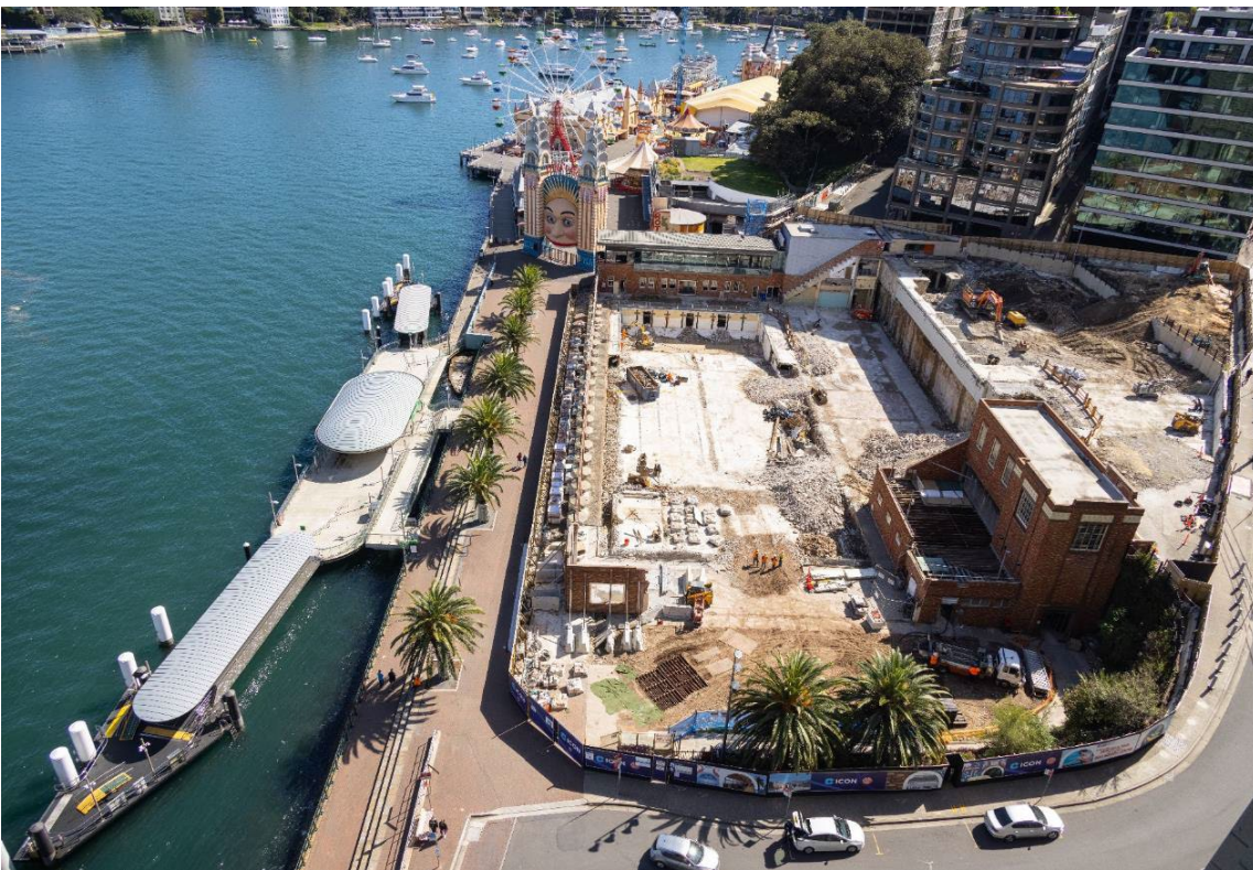
Under Construction - North Sydney Olympic Pool Redevelopment – commenced March 2021- Scheduled for completion late 2023. ($64million)
