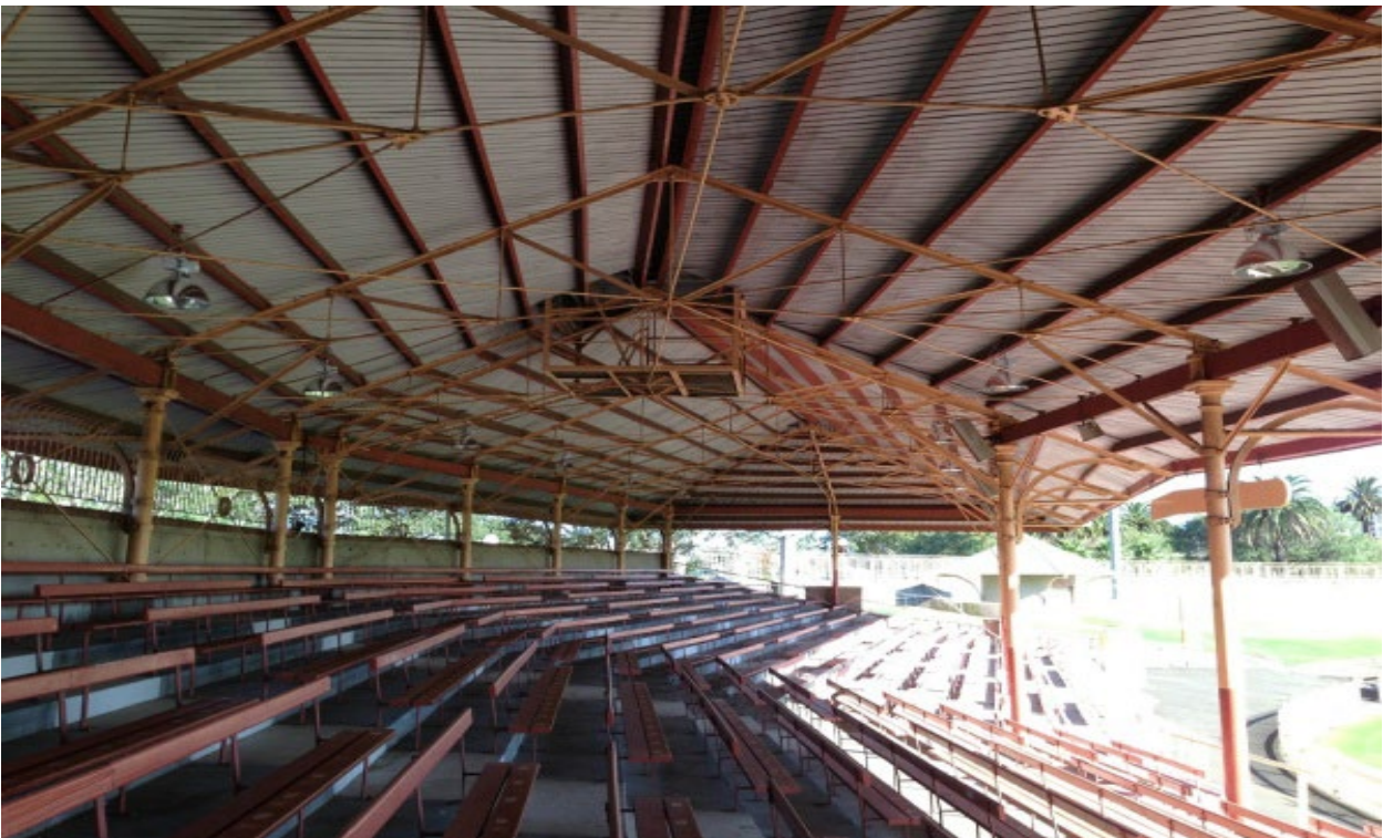
Councils Property team organise and undertake significant maintenance works on North Sydney Oval including roof replacement of the grandstands- painting and structural repairs each year
