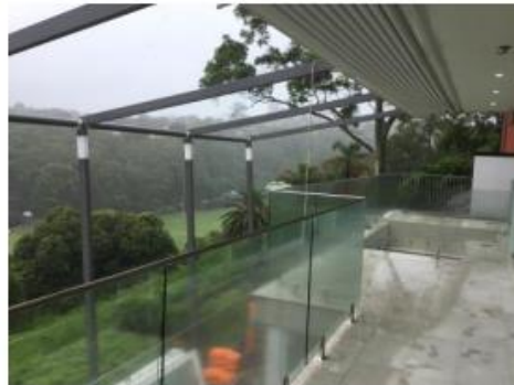
Basement Level Lighting installed in support posts Looking South
