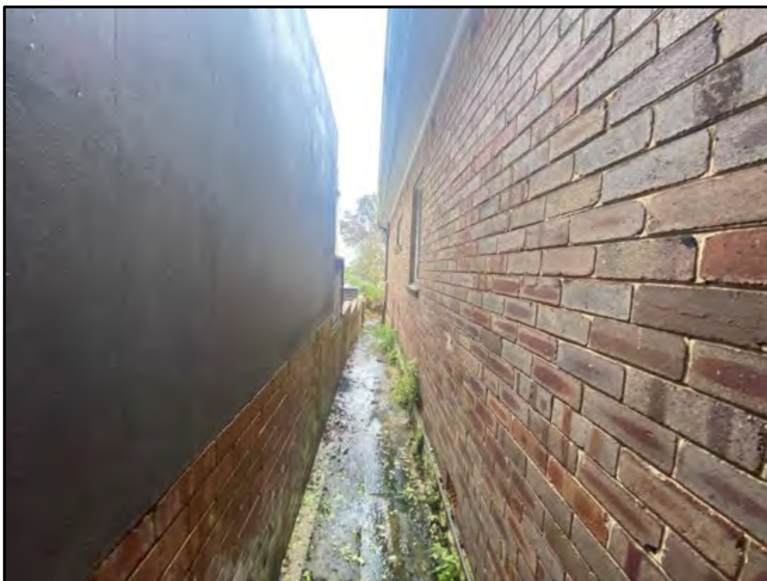
Figure 20: Existing paved path and fencing/walls along southern side setback – view towards Thomas Street
