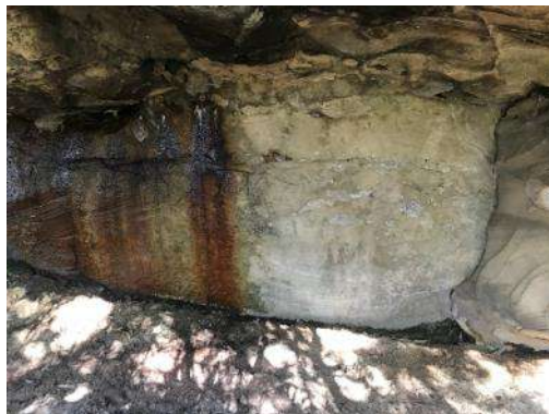
Moisture in shelter, Castle Cove
