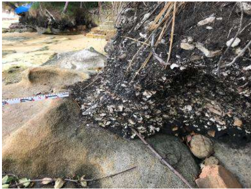
Coastal erosion, Northbridge
