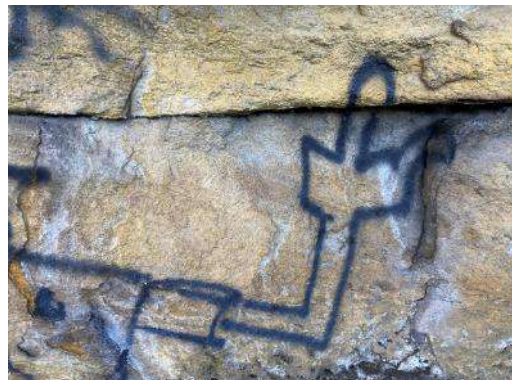
Graffiti inspection, Lindfield
