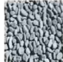
6 Pebble ballast roof
