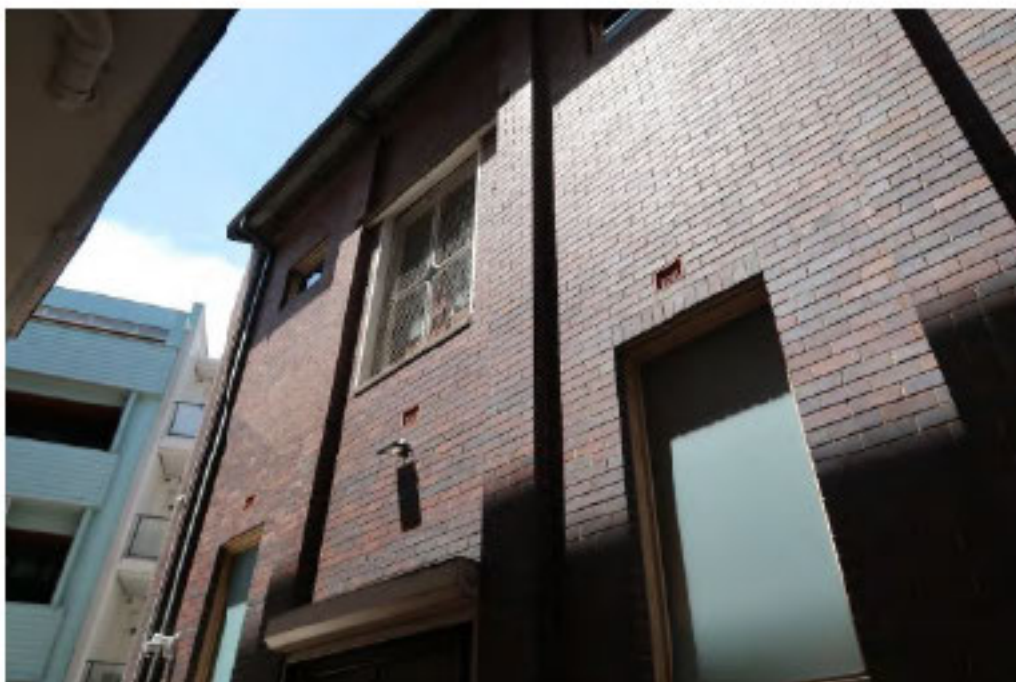
Figure 16: First floor exterior of the northern facade of the subject site, the proposed location of the gallery addition. The existing first floor opening to be utilised within the proposed works visible centrally (Source: NBR)
