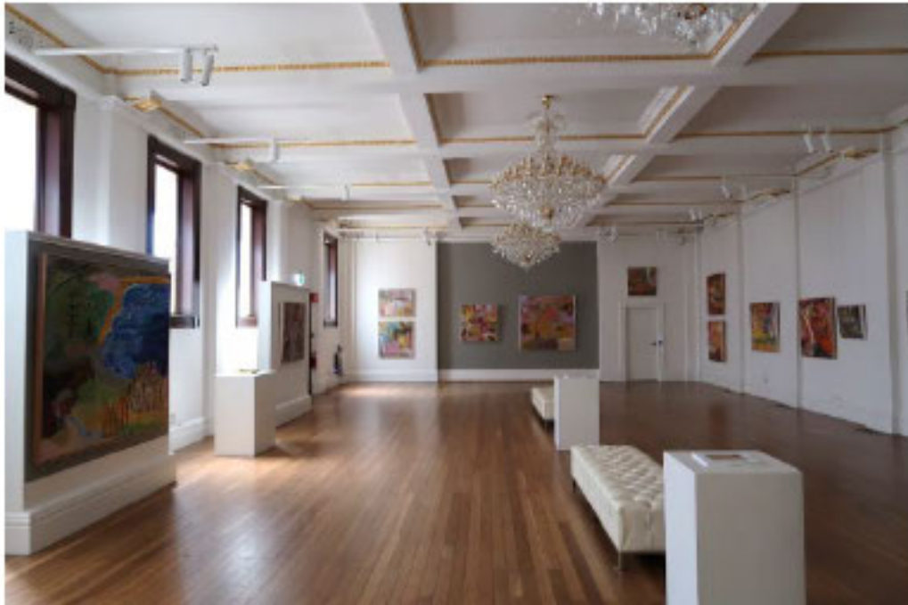
Figure 19: Main Hall on the ground floor of the site, details of coffered ceilings and rendered masonry piers visible, view looking east (Source: NBR)
