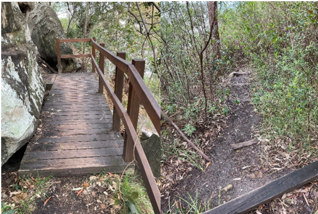
Above left: Raised timber boardwalk with decayed decking timbers
