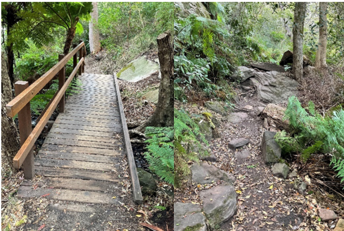
Above left: Raised boardwalk with decayed decking timbers
