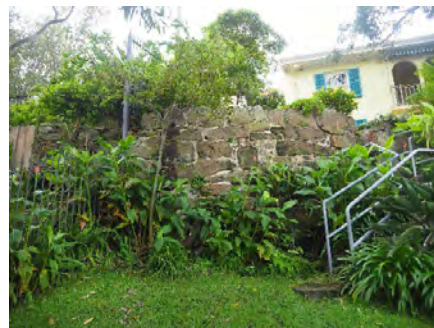
Figure 3. 34: Sandstone retaining along northern side of the terrace area above. Note metal handrails for central steps.
