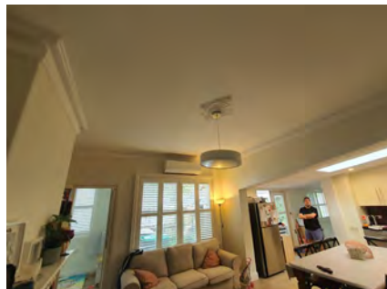
Figure 2. 26: Original cornices and ceiling rose (damaged) to living room.
