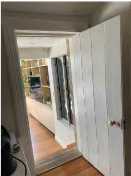
Rear ledged door. Battens too wide for 1860s.
