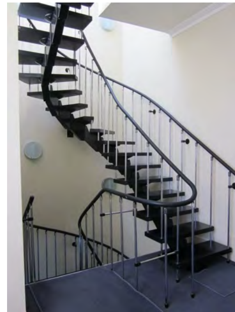
Existing staircase is non-compliant
