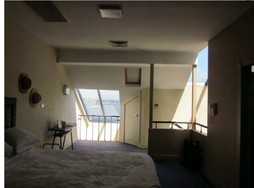
Attic storey with west facing glazing and no openable windows
