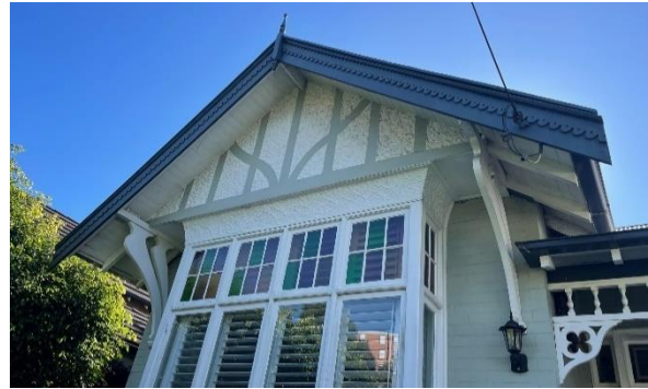
Figure 5.32 View showing a detail of the gable end, with decorative half timbering, roughcast finish, timber brackets and bargeboards and finial and pressed metal cladding.
