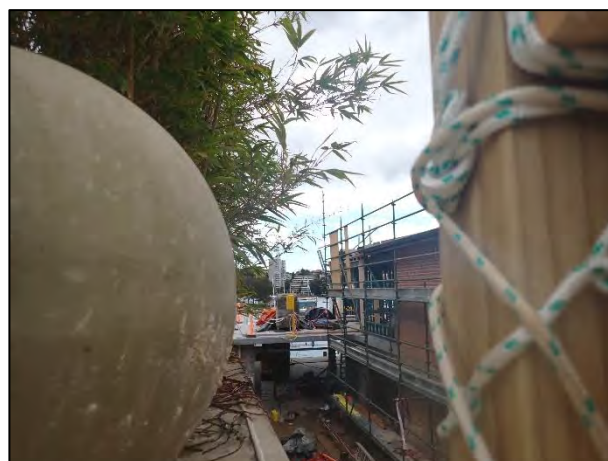
Figure 10. View of the eastern side elevation from the Elamang Avenue street level.
