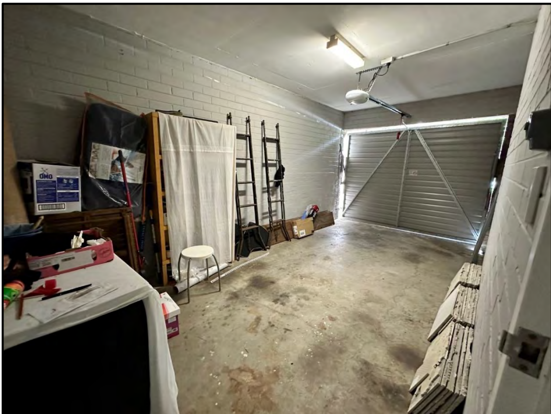
Figure 13: Internal view of garage of Unit 6 – to be converted into a multi-media room
