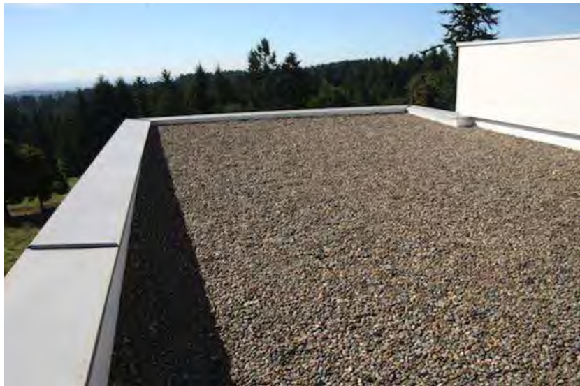
Pebble ballast roof
