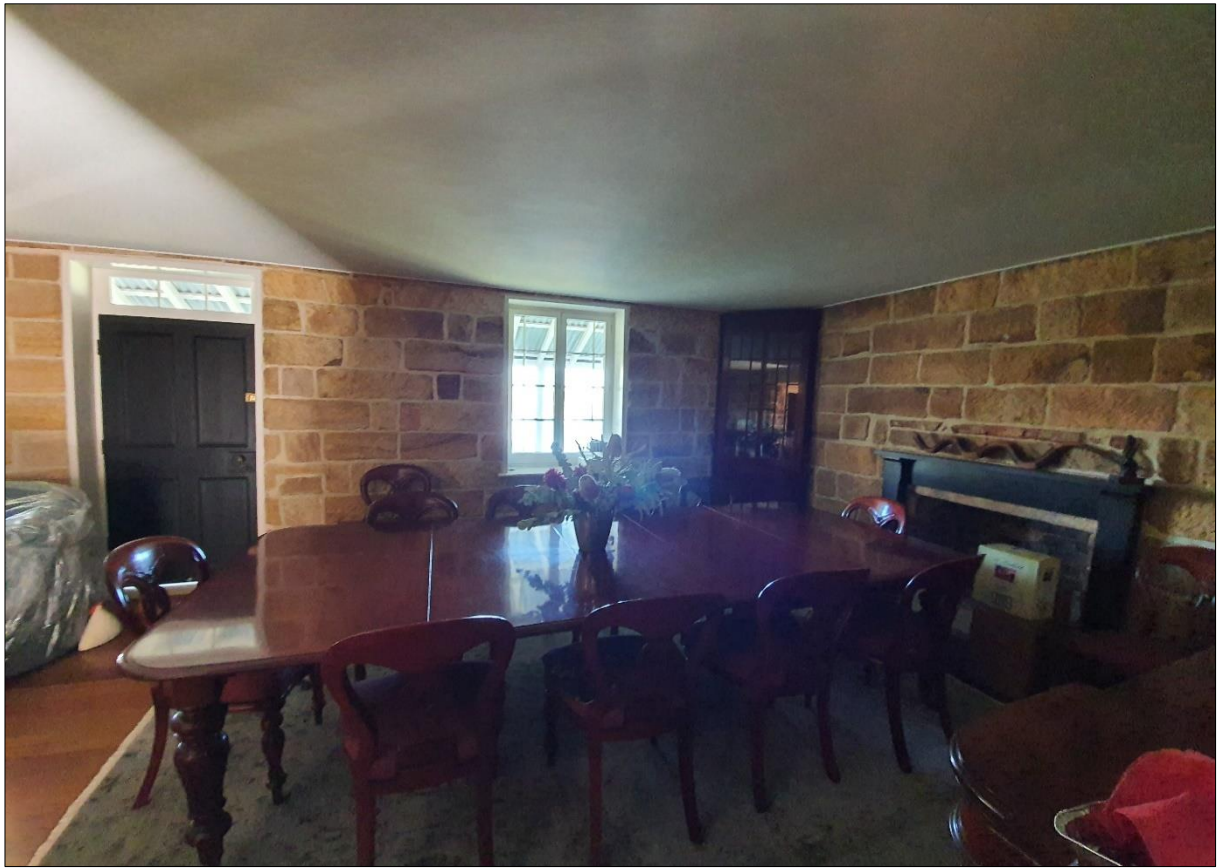
Figure 9t: Photo taken of Ground Floor Dining Area during June 2023 site inspection
