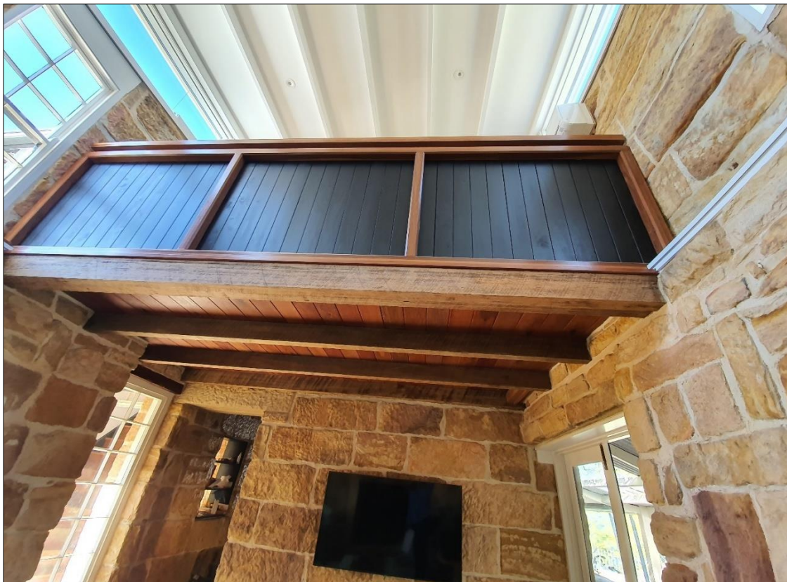
Figure 9n: View from Family Room to Mezzanine level above created through unauthorized works
