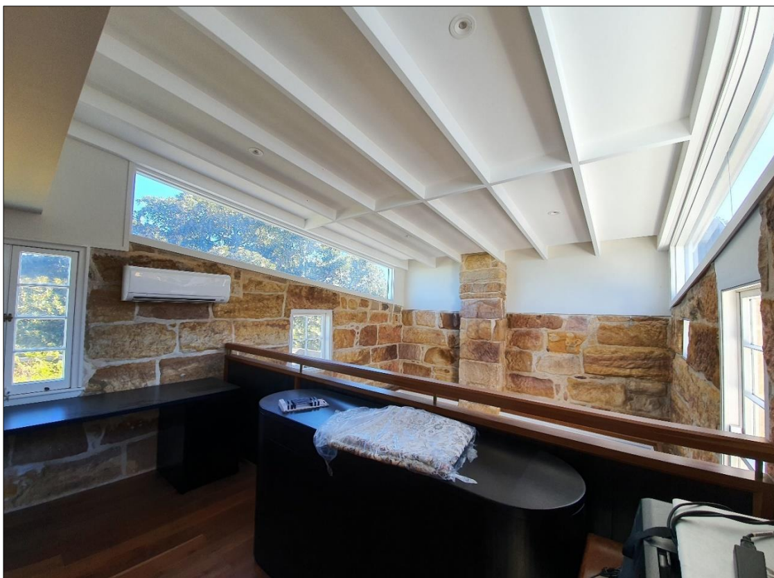
Figure 9l: View towards Bedroom 3 with unauthorised works that created a void and mezzanine
