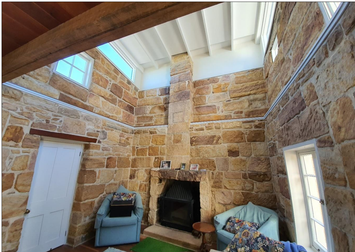
Figure 9v: Photo of Family Room on site inspection June 2023 (with ceiling and cornices removed)
