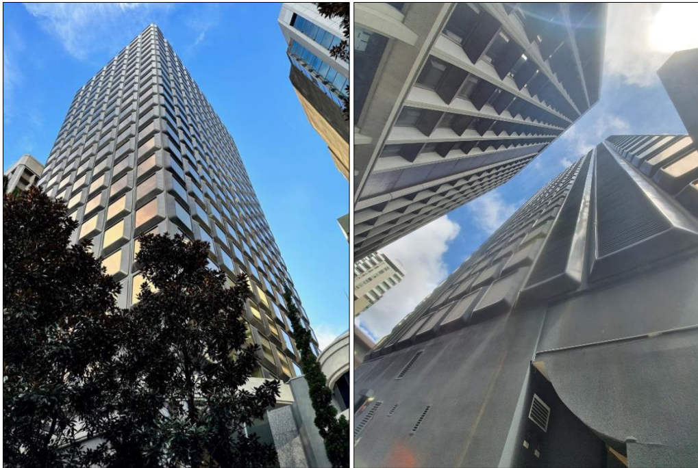
Figure 7c (left): SW view of existing building; Figure 7d (right): Northern elevation of building with 4 columns of existing vertical louvers
