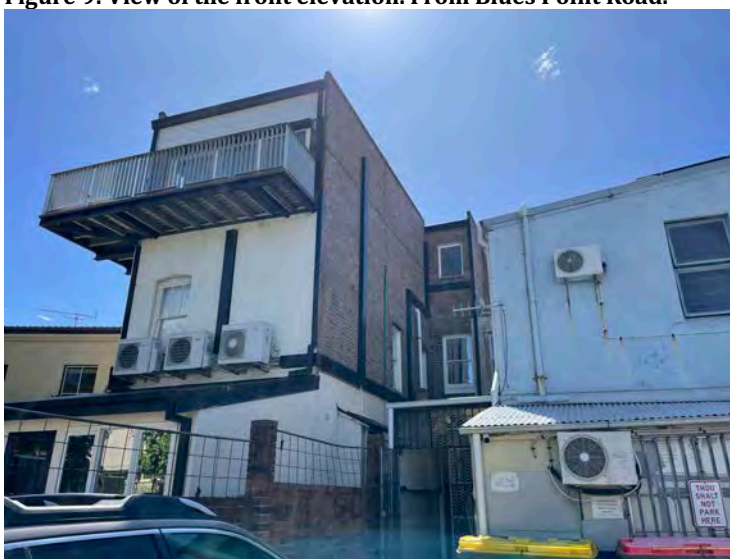
Figure 10: Looking south west towards the north and east elevations of the rear wing
