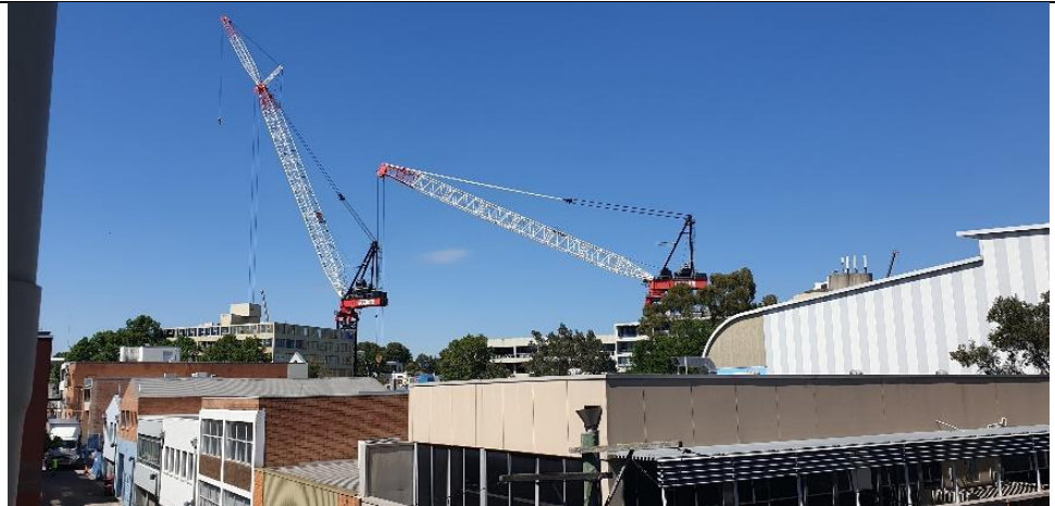
Figure 11: Construction of Crows Nest Metro Station, 80m west, image taken from the roof of the site.
