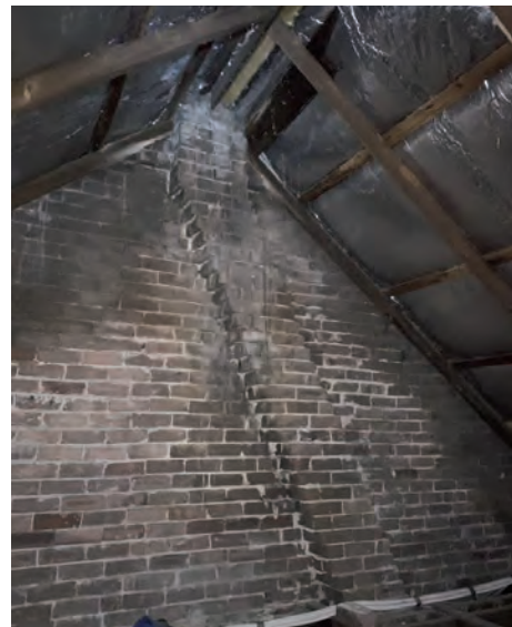
Figure 3.13 Note retrofitted sarking and new ridgeboard denoting roof repairs conducted recently.
