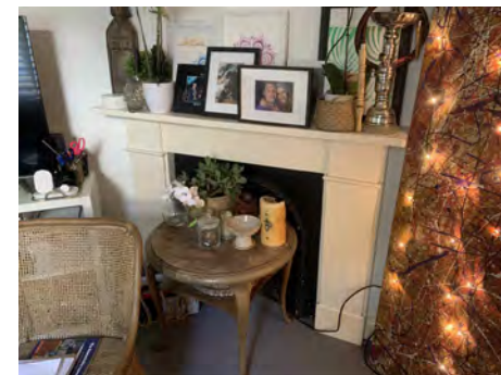
LIVING ROOM FIREPLACE TO BE DEMOLISHED TO PERMIT EXTENSION OF EXISTING HALLWAY ALONG THE PARTY WALL TO THE PROPOSED ADDITIONS.
