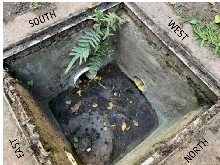
EXISTING STORMWATER PIT CLOSE TO BOUNDARY BETWEEN LOTS 141 & 142.
