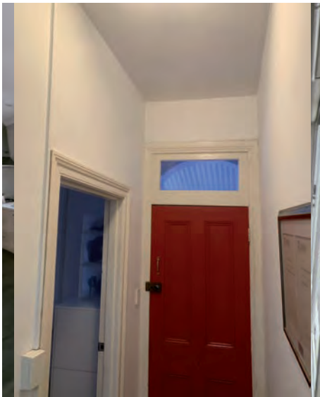
Figure 3.8 main hallway looking towards front door. note lack of decorative cornicing and ceilings.
