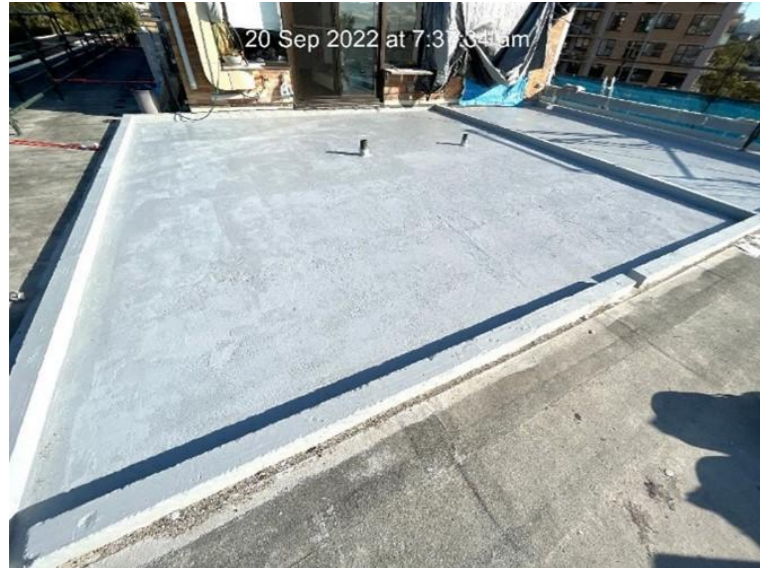
EPOXY APPLIED TO SUNROOM AND TERRACE AREAS, SCREED AND FALL WAS CREATED (20 SEP 2022)
