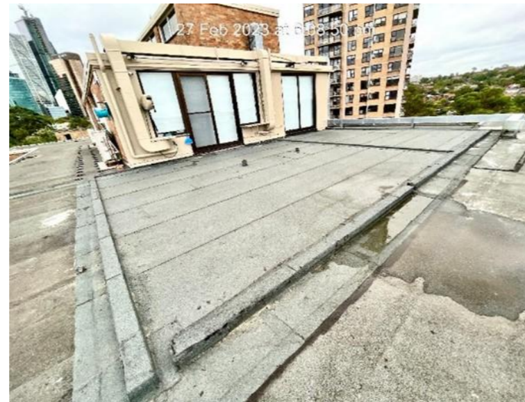
WATERPROOFING ON THE EXISTING ROOF SLAB AND SUNROOM DOORWAY INSTALLATION COMPLETED (27 FEB 2023) - SOUTH EAST VIEW
