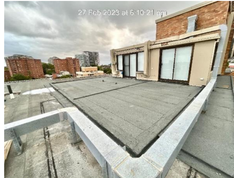
WATERPROOFING ON THE EXISTING ROOF SLAB AND SUNROOM DOORWAY INSTALLATION COMPLETED (27 FEB 2023) NORTH EAST VIEW
