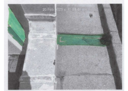
NORTHERN PATHWAY: DRAINING OUTLET - PIT DRAINS IN A PIPE ALONG THE WALL
