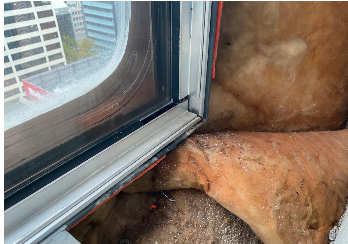
Evidence of water ingress and deterioration of substrate
