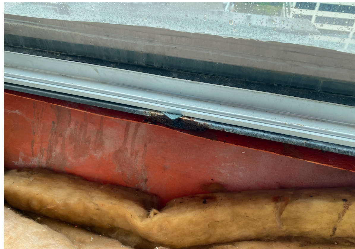
Corrosion of fixings
