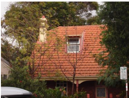
Figure B-13.24: The simple roof form of Federation and Interwar houses can be sympathetically altered using dormers that form gablets.
