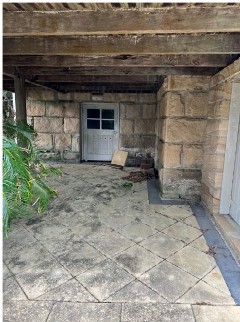
Figure 28 - Sandstone base course below the later timber verandah. Early door providing access to the sub floor space.
