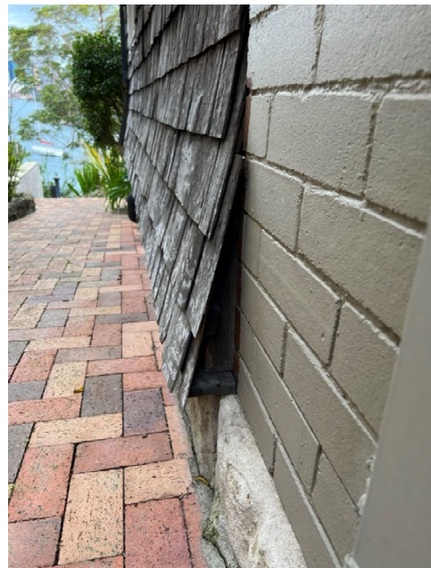
Figure 29 - Traditional 'bell bottom' or 'cat slide' detail to the edge of the wall shingles.
