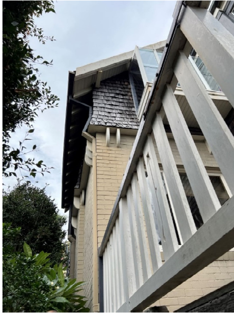
Figure 30 - Detail image showing the addition of the timber verandah, along with the upper later 'glass box' view window in the timber shingled wall.
