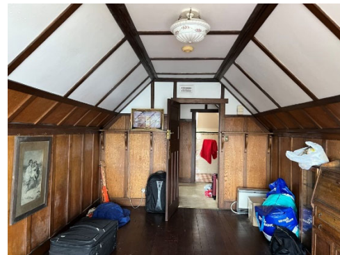
Figure 38 - View back towards the entry landing at the top of the stair leading to the Attic.
