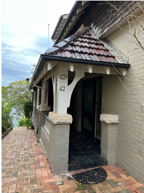
Figure 26 - View of the front entry with painted brickwork, joinery and later door joinery just visible. The original joinery, shown in figure 24 is out of site.
