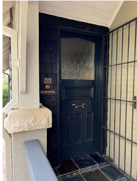
Figure 27 - original timber joinery door and framing. The threshold and original tiling has been lost.
