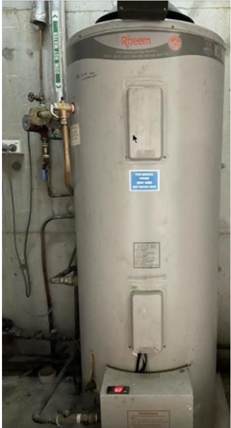
Old gas boiler
