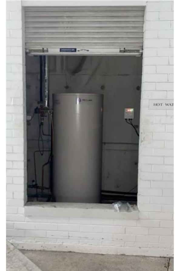
Tank for heat pump
