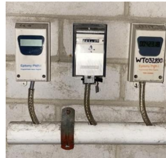
Legacy hot water meters with digital display
