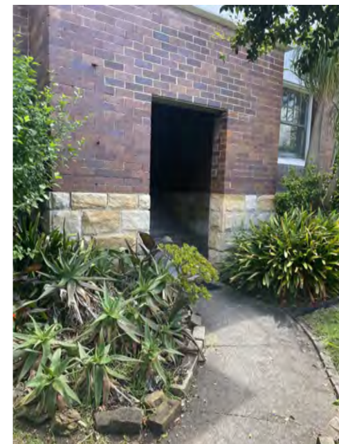
9. Widen front entry for dual access with recycled bricks 10. Repoint sandstone base 11. Restore front path and garden edge with recycled bricks
