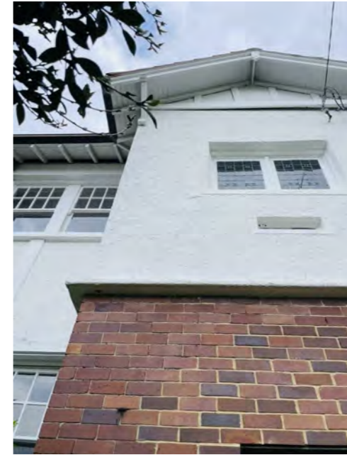
1. Retain and restore bell cast rail 2. Retain and restore white stucco 3. Repoint existing brickwork 4. Retain lead light window (new infill window behind) 5. Restore 'St Martin's' lightbox sign
