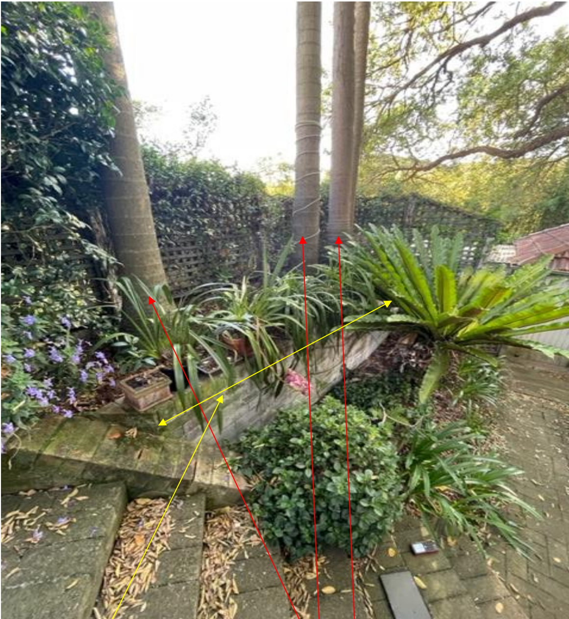
Photo A: The existing wall may be providing support for Trees 5,6 and 7 and is recommended to be retained and the area filled around. See section 7 and 8.2 for discussion.
