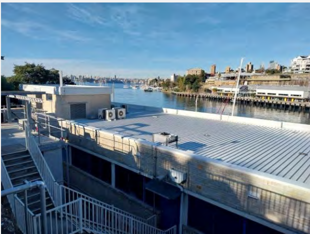
PHOTOGRAPH 2-8 VIEW OF THE ROOF OF THE ADMINISTRATION BUILDING FROM THE UPPER CARPARK (ERM 2023)
