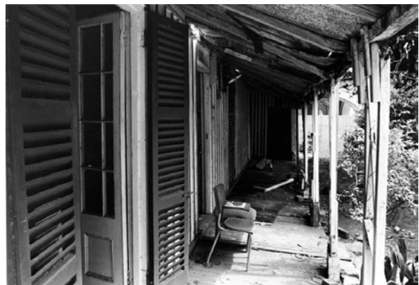
Figure 2. 39: View of the front (east) verandah of Don Bank prior to restoration. Source: Stanton Library
