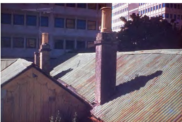
Figure 2. 42: A photograph by Beryl Graham of the roof materials of Don Bank in February 1974. Source: Stanton Library (CT11/34)
