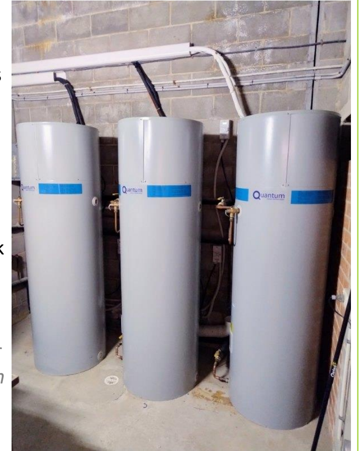
New tanks in hot water room
