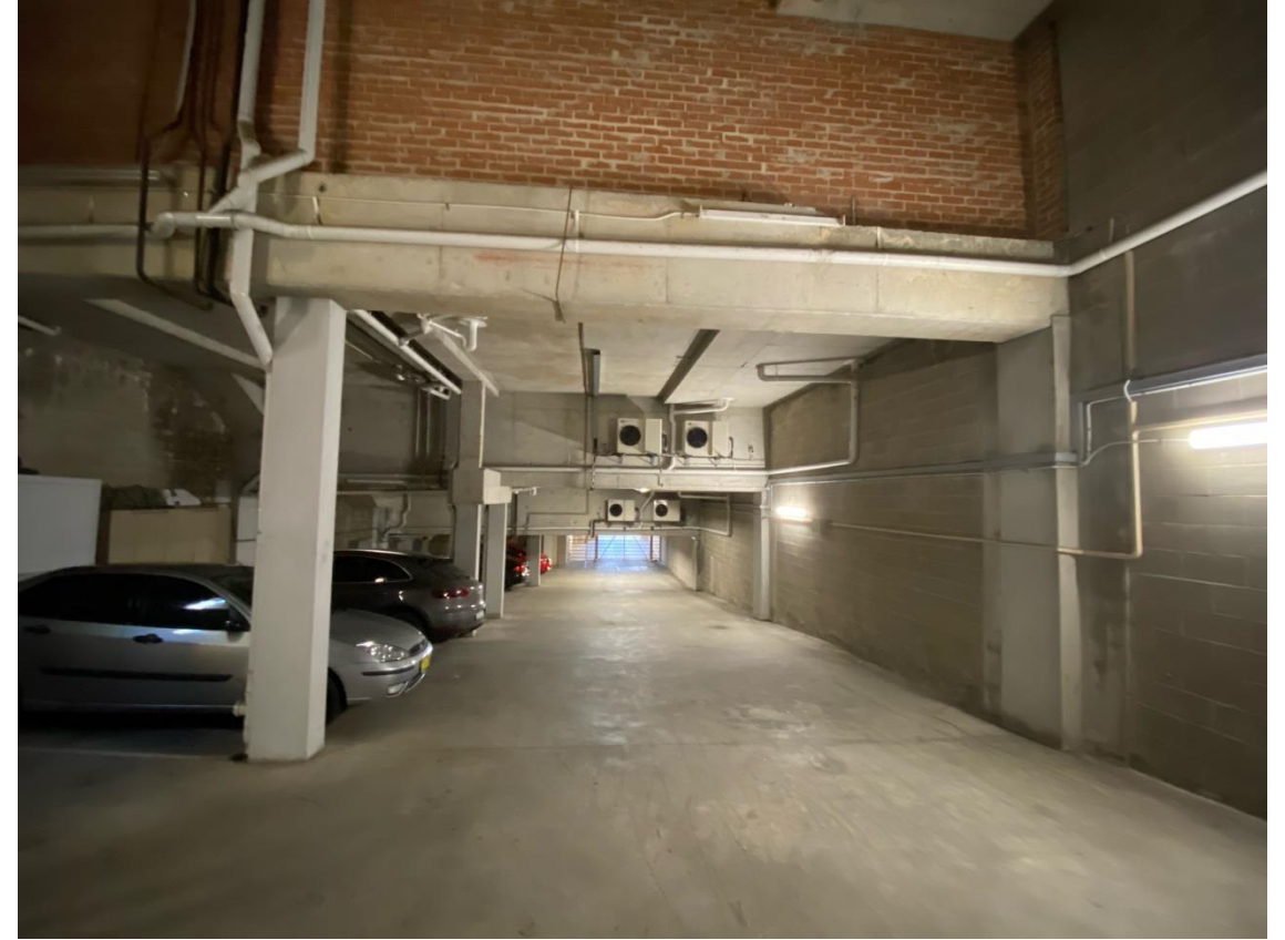
Existing split air conditioning units mounted in the carpark area push warm air into the carpark, which improves performance of the heat pumps
