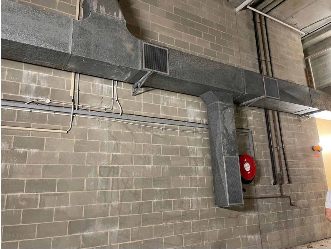
Carpark wall adjacent to hot water plant room has space to install the heat pump compressors
