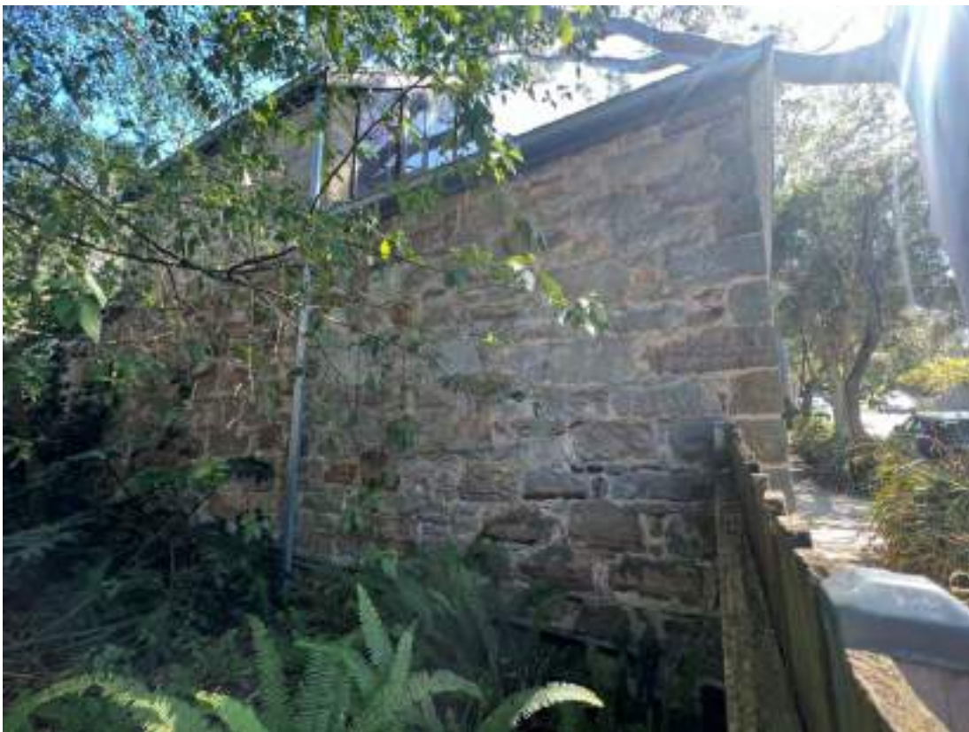
South elevation (over adjacent fence). Coursed rubble. Poor cementitious repointing is evident. The rear 1980s extended section is not visible from the public realm and would have to be viewed from the rear garden of 19 Clifton Street, which runs through to Euroka Street.
