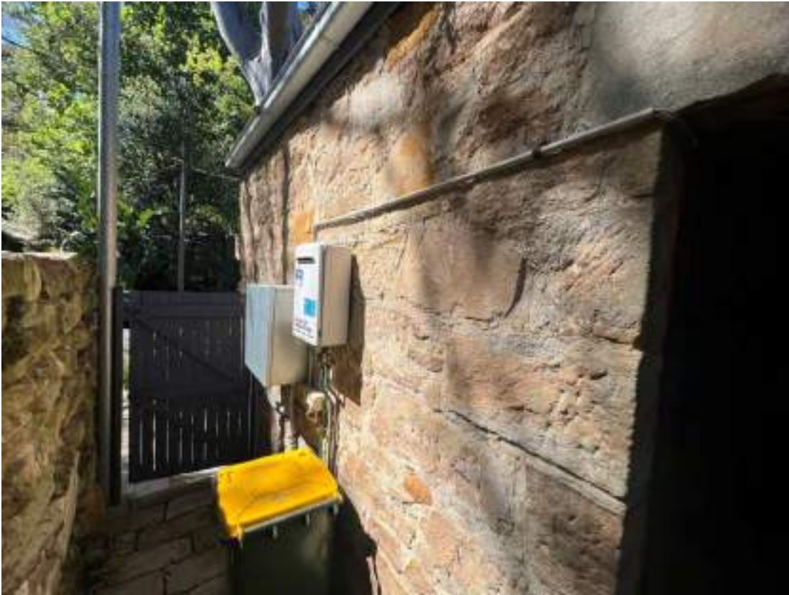
Front portion of the north elevation, facing Eureka Street. Cementitious mortar. Some blocks show signs of what appears to be exfoliation.
