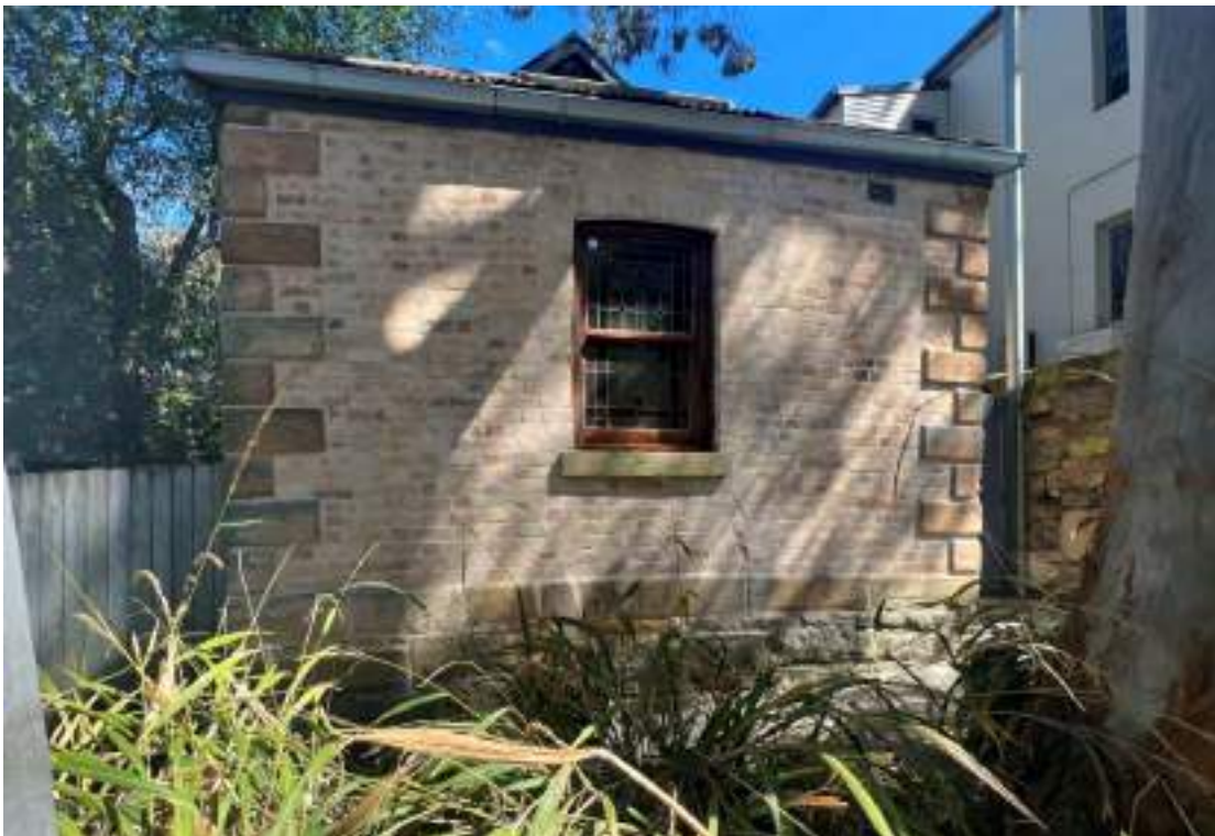
Close-up of the façade with sandstone plinth and quoining and soft brick (Flemish bond) to the body of the wall. Some sandstone blocks in the plinth display signs of fretting.
