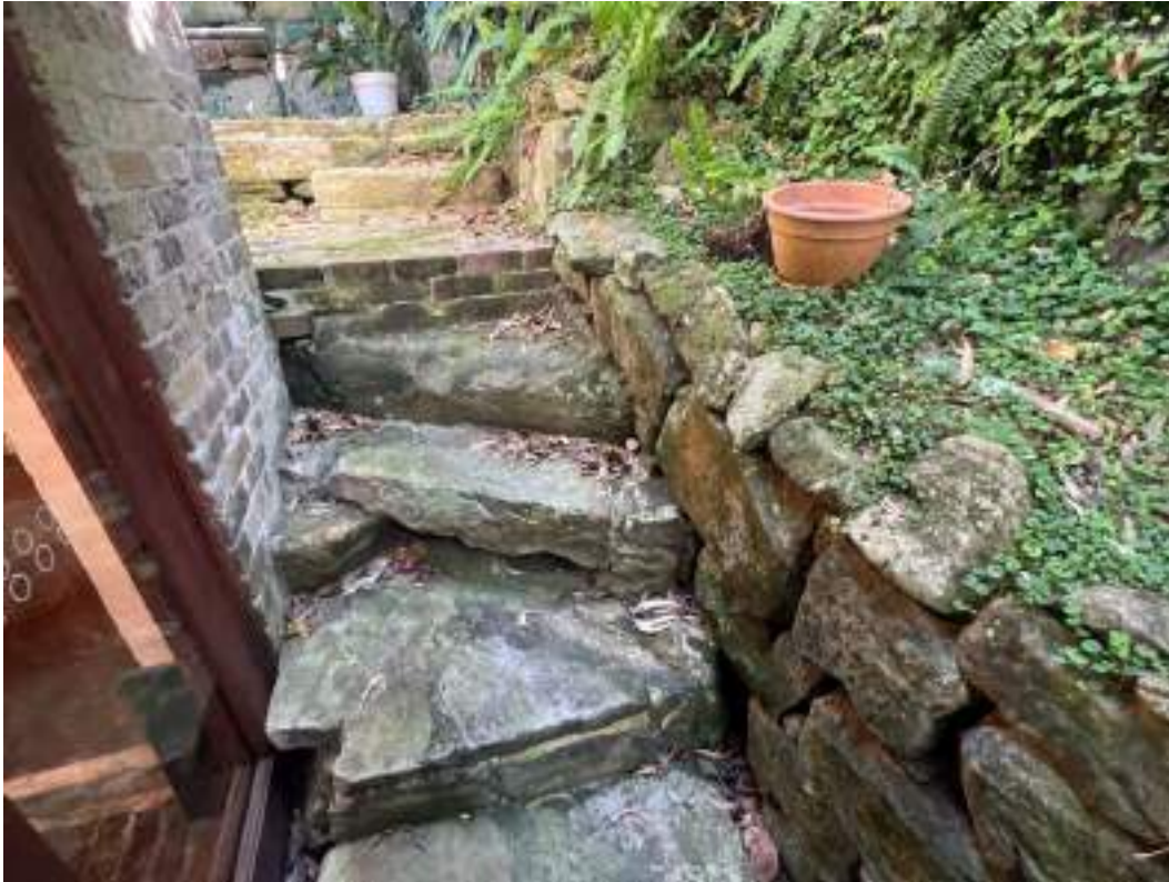
Roughly shaped sandstone steps and retaining wall/rock shelf—northwest corner of the ground floor.
