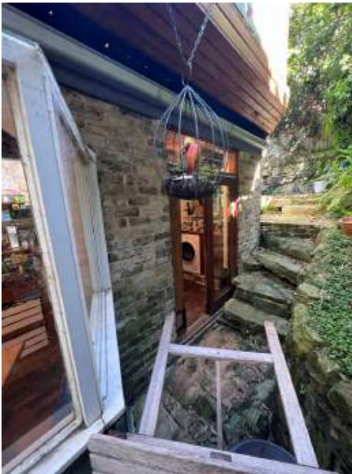
Rear part of the north elevation, past bay window. Brick with deck above.
