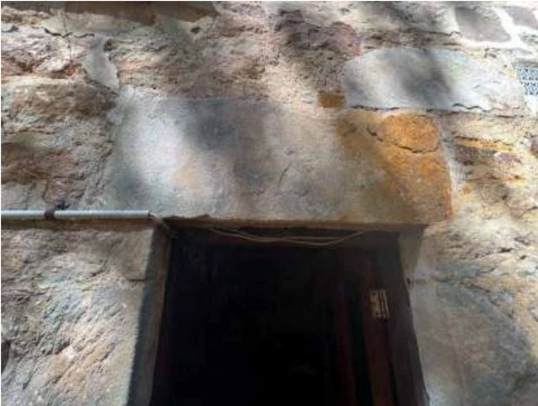
Close-up of 'massive' lintel (see following image). Note brown staining/discolouration in top right, cause unclear.
