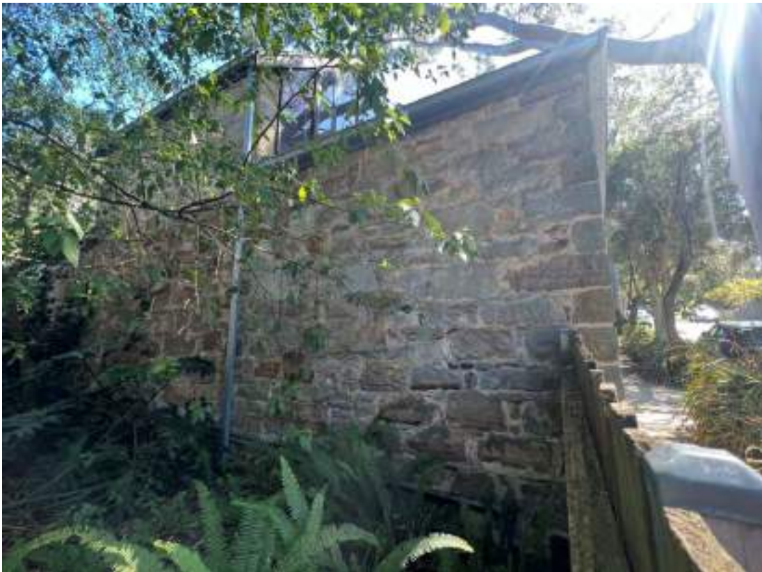
South elevation (over adjacent fence). Coursed rubble. Poor cementitious repointing is evident. The rear 1980s extended section is not visible from the public realm and would have to be viewed from the rear garden of 19 Clifton Street, which runs through to Euroka Street.
