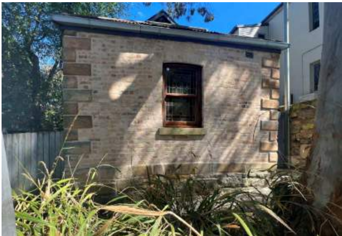
Close-up of the façade with sandstone plinth and quoining and soft brick (Flemish bond) to the body of the wall. Some sandstone blocks in the plinth display signs of fretting.
