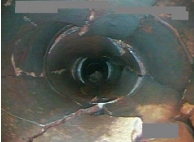
Pipe in very poor condition
