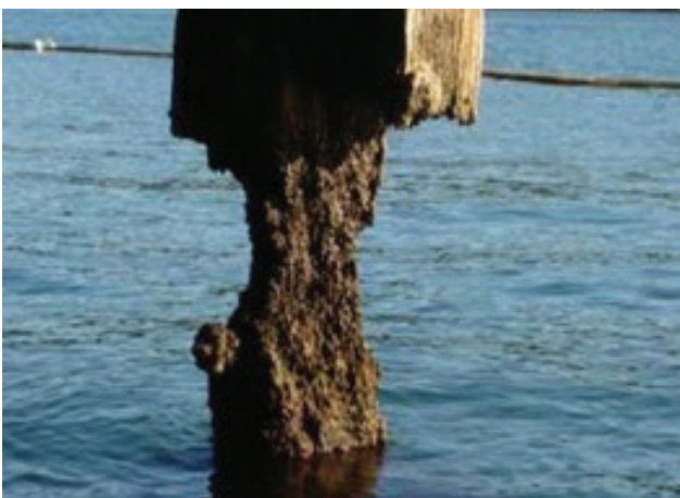
Pile in very poor condition
