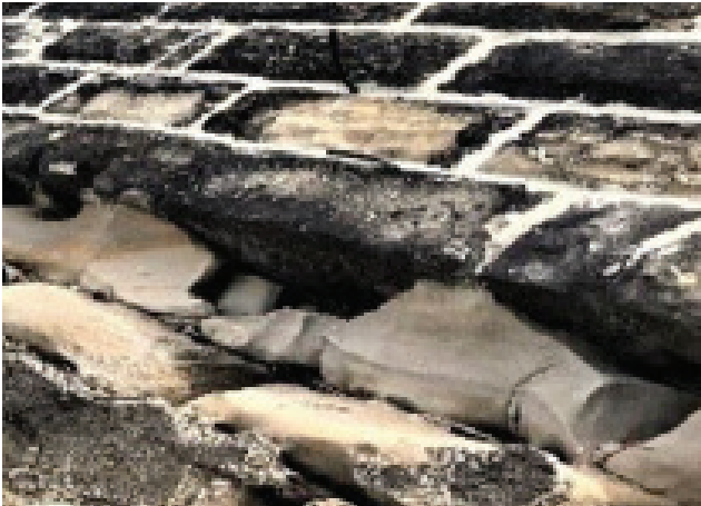
Blocks missing and eroded
