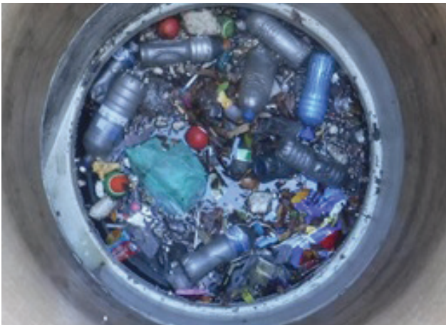
GPT prior to cleaning
