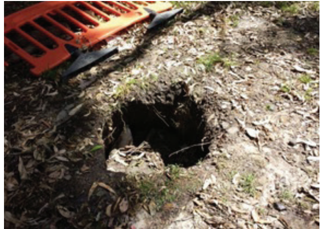
Sink hole in reserve near pipe
