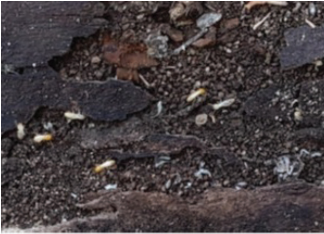
Termites found in timber marine structure
