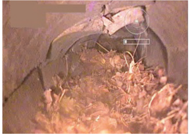
Pipe in very poor condition
