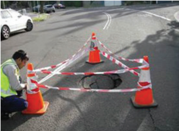
Sink hole in road near pipe
