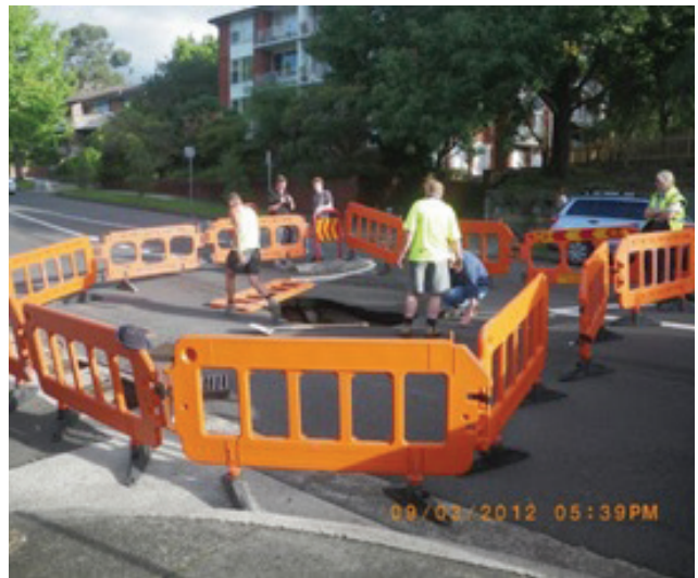
Sink hole in road near pipe
