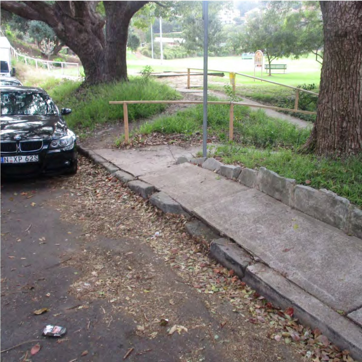
Examples of failed Kerb and Gutter in the North Sydney LGA
