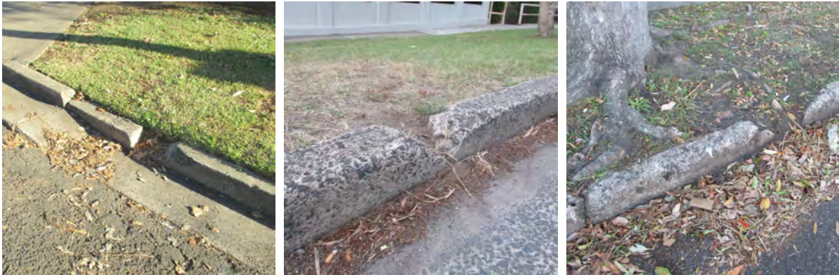
Examples of failed and failing Kerb and Gutter in the North Sydney LGA
