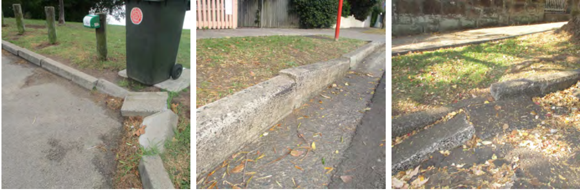
Examples of failed Kerb and Gutter in the North Sydney LGA
