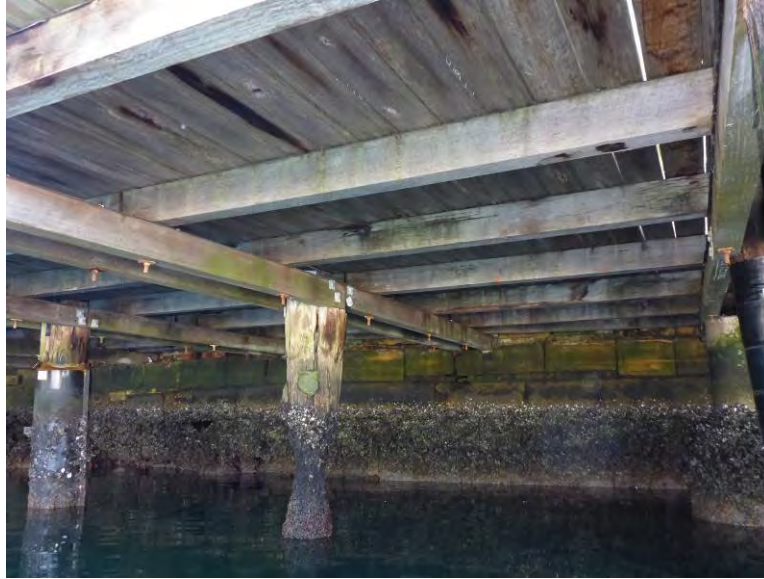
Examples failing timber piles – Wondakiah wharf
