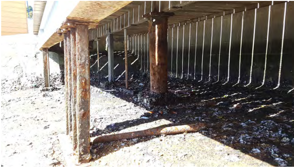
Examples failing steel piles – Boatbuilders Walk Bridge
