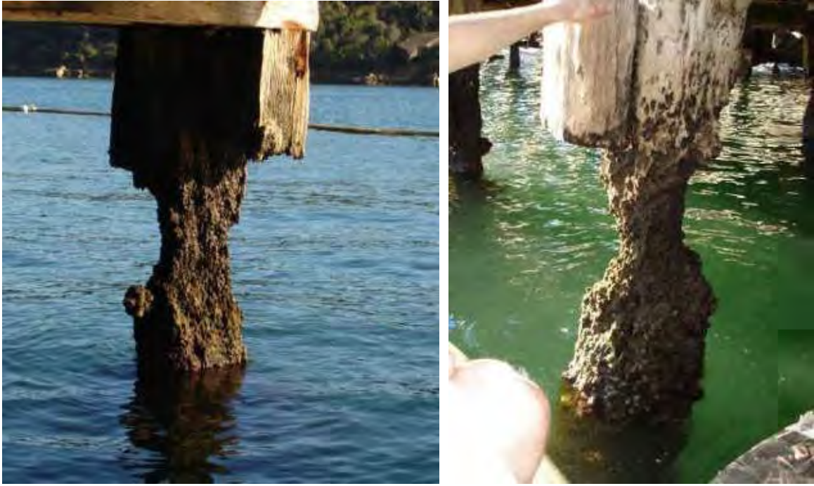
Examples of piles in very poor condition
