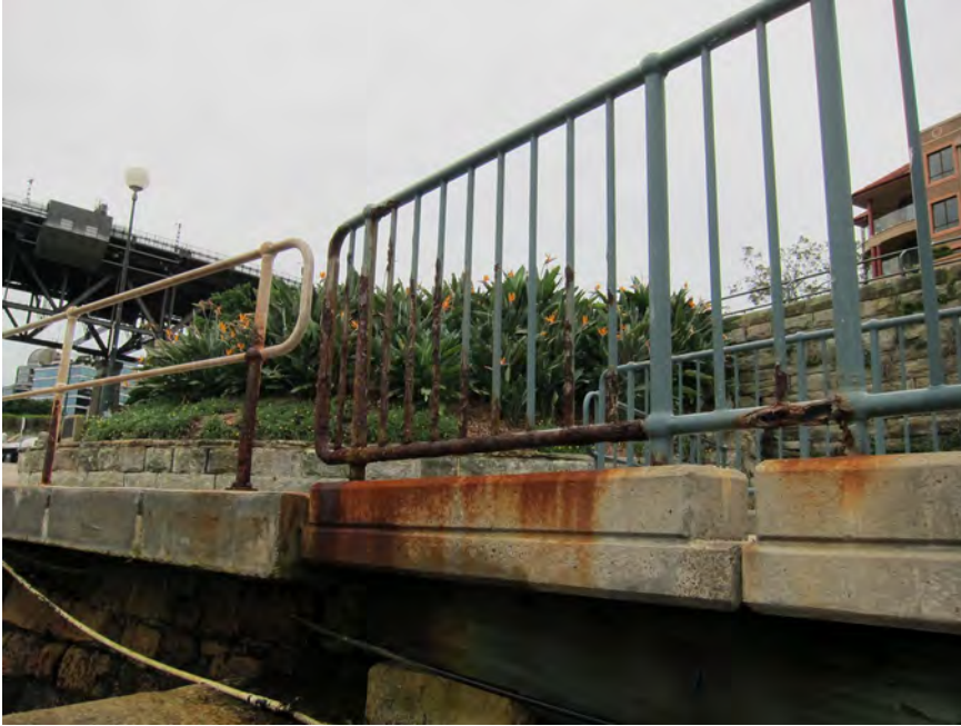
Examples corroding fence – Jefferys Street Bridge
