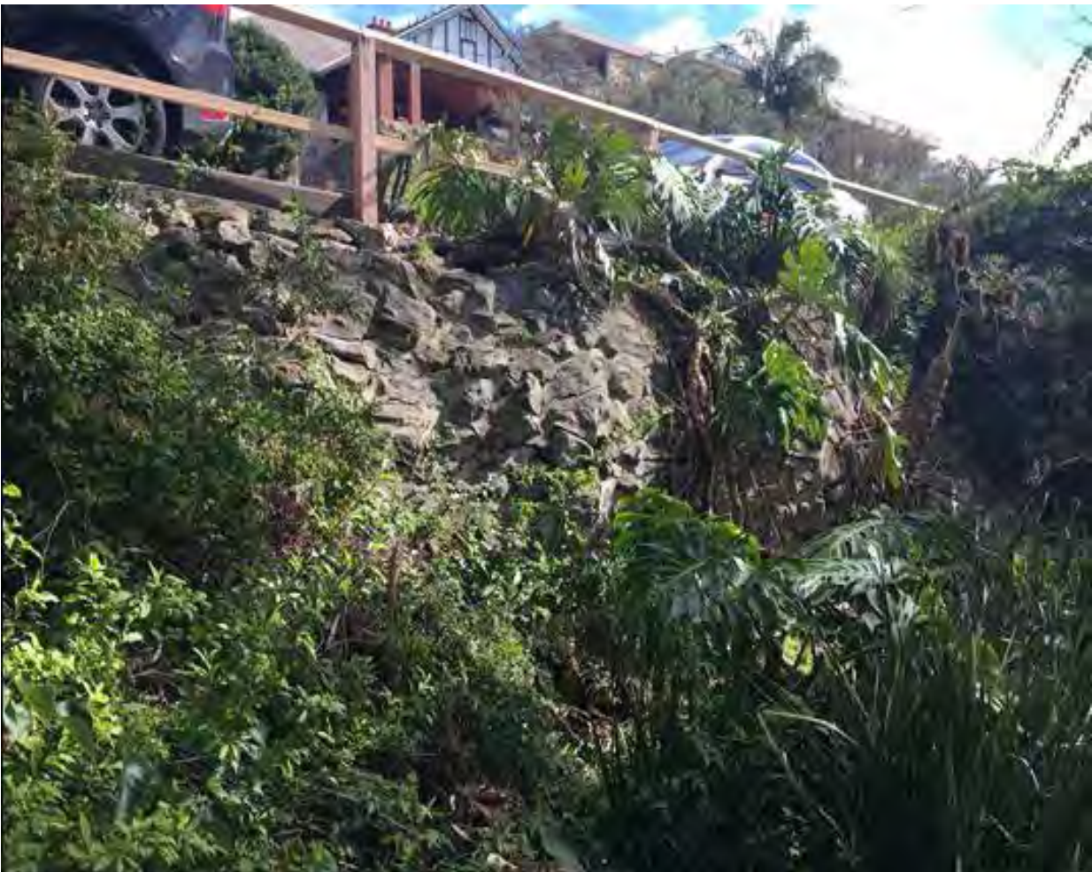
Examples of failed and failing retaining walls in the North Sydney LGA
