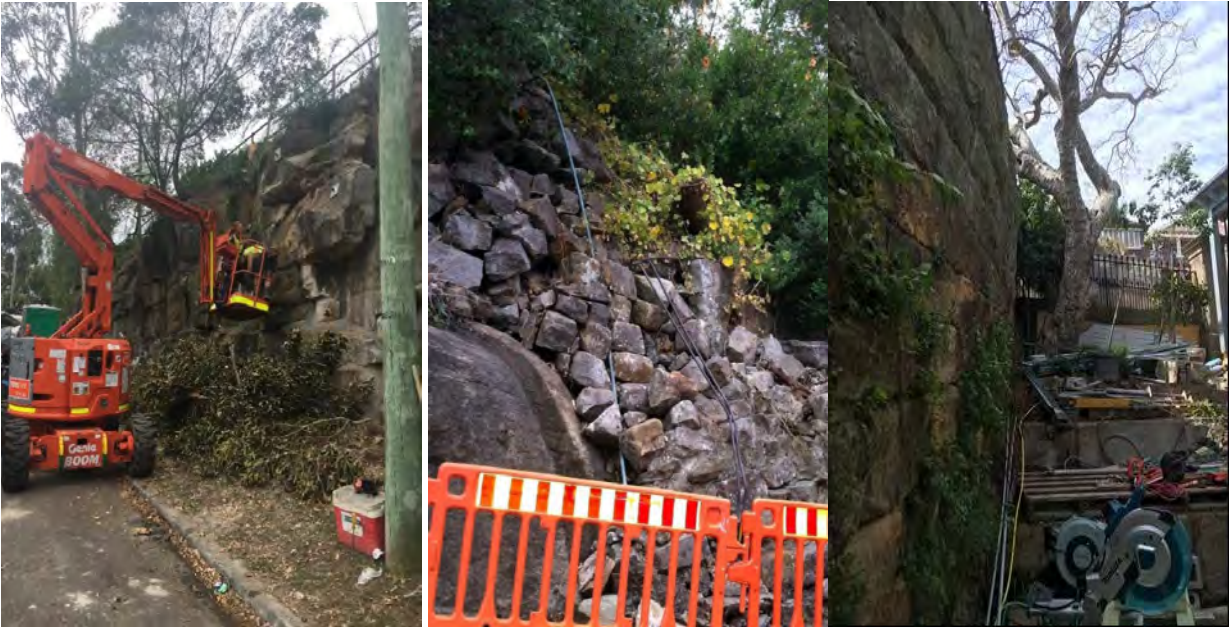
Examples of failed and failing retaining walls in the North Sydney LGA
