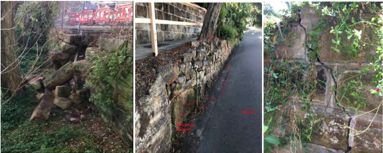
Examples of failed and failing retaining walls in the North Sydney LGA
