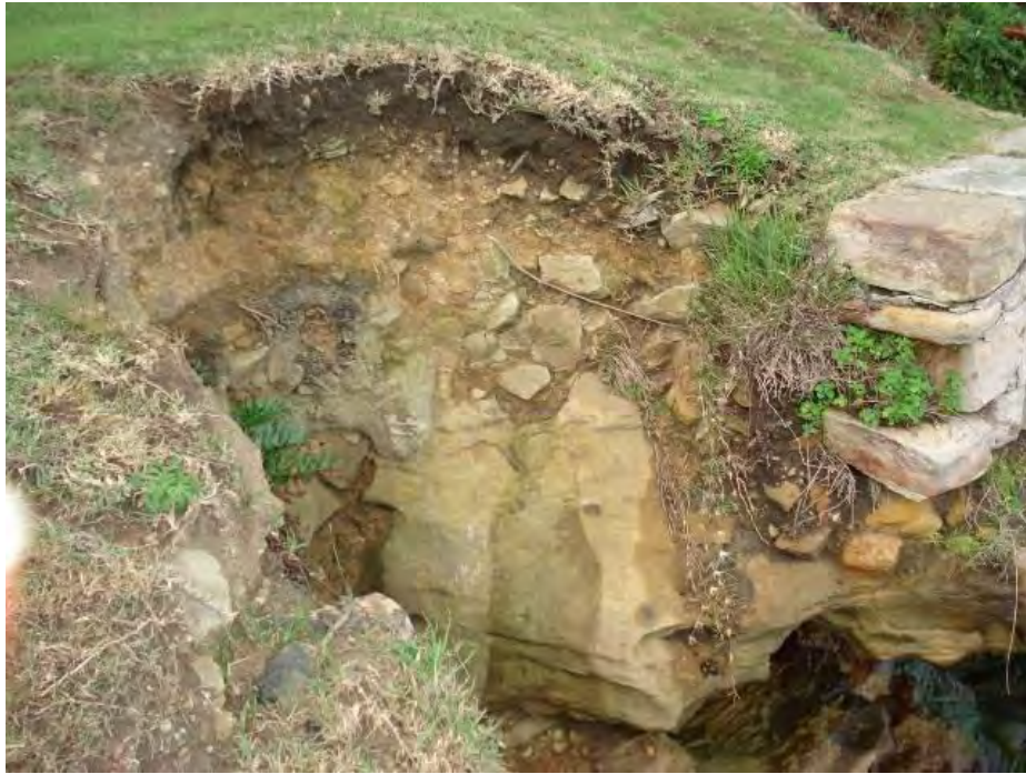
Examples of failed and failing seawalls in the North Sydney LGA – Cremorne Point
