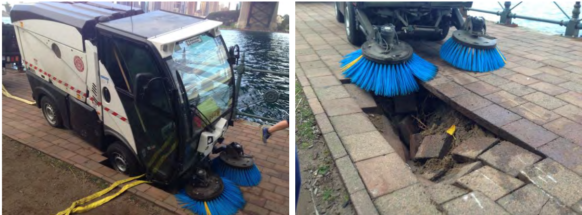
Examples of failed and failing seawalls in the North Sydney LGA – Bradfield Park
