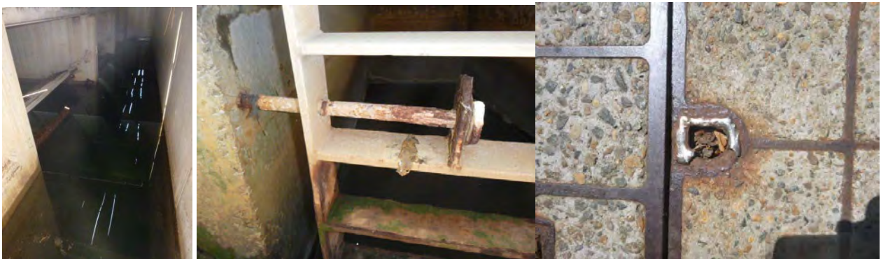
Trashracks is bent over and there is a lot of rust. Exclusion bars are rusting – lifting points are rusting due to the corrosive environment
