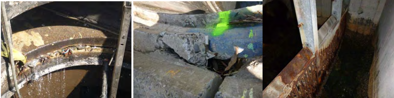
Corrosion and structural damage to a number of pits
