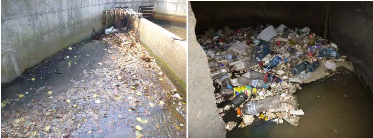
Sediment and trash build up in front of the weir and in pits generally – low capacity.
