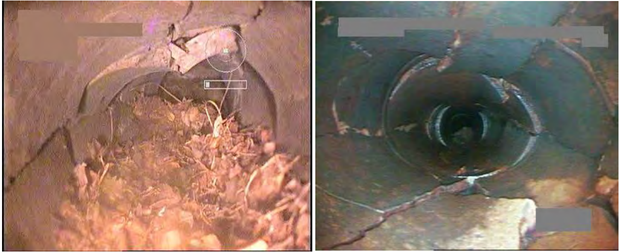
Stormwater Pipes in very poor condition – collapsed and blocked
