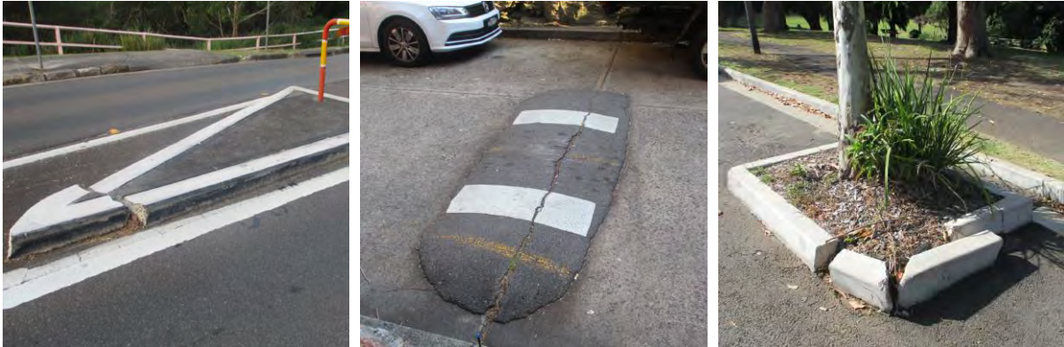
Examples of failed and failing Traffic Facilities in the North Sydney LGA
