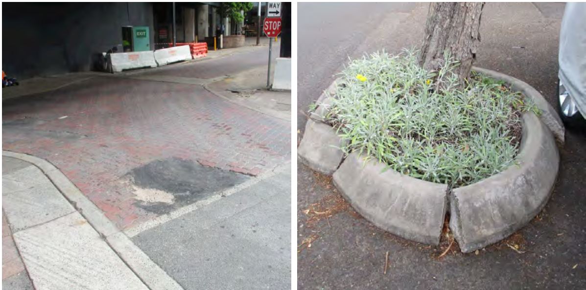
Examples of failed Traffic Facilities in the North Sydney LGA
